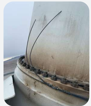
Figure 1: Level 4 hose damage noted on turbine pitch bearing.
