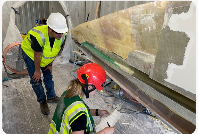
Figure 2: ONYX's Megan Rotondo inspecting blade damage for a root cause analysis
