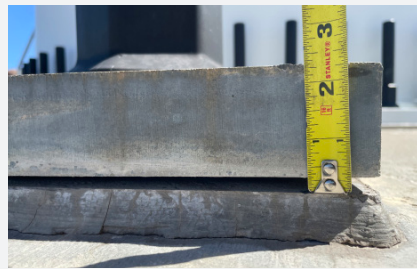
Figure 1: Gap in bearing plate
